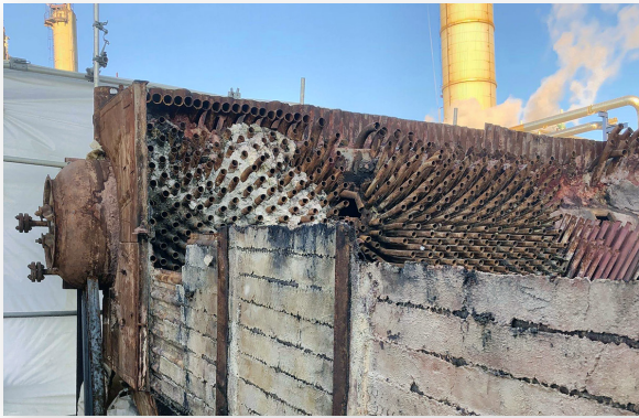
The construction team disassembled the existing unit that was negatively impacting the plant's production.
