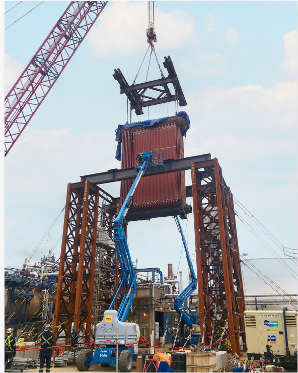
B&W's construction team built the replacement boiler in a jig concurrent with the demolition of the existing unit to minimize the plant's outage time.
